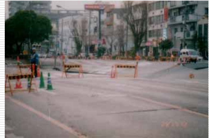
Subsidence of Road Surface
