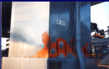
Damage Cases in Steel Bridge Piers In the 1995 Hyogo-ken Nanbu Earthquake
