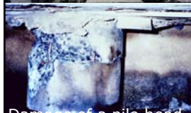
Damage of a pile head
