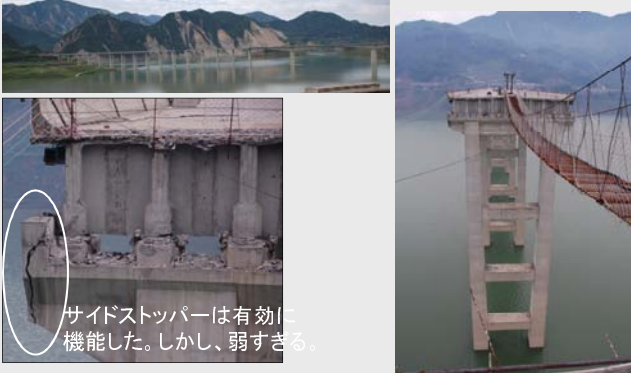
Damage Resulted from Ground Motion Effect 2008 Wenchuan, China, Earthquake
