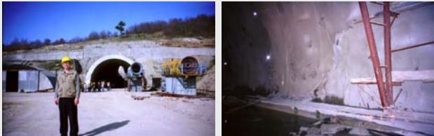
Damage of a tunnel 1999 Bolu, Turkey earthquake
